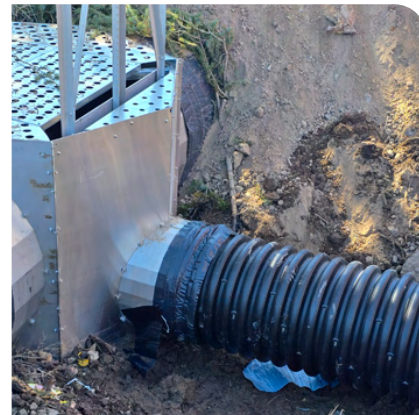
SmoothCorr pipe connects to the stainless steel control structure which manages water flow and diversion.
